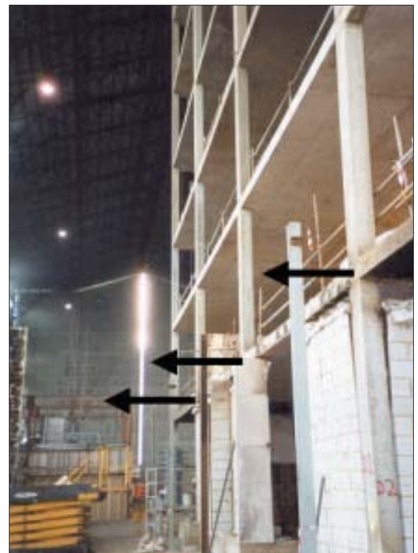
Fig 11. Picture showing lateral movement of external columns following a fire test on the Cardington Concrete Building
