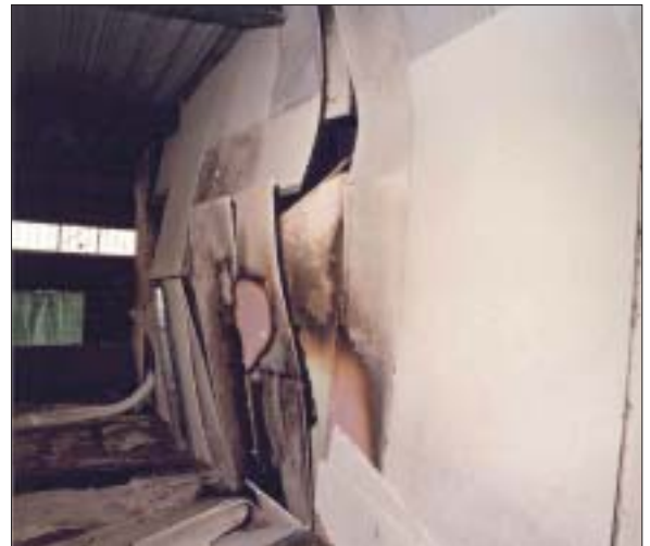
Fig 4. Deformation of structure causing failure of compartment wall
