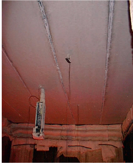
Figure 24 Underside of slab B post-test
