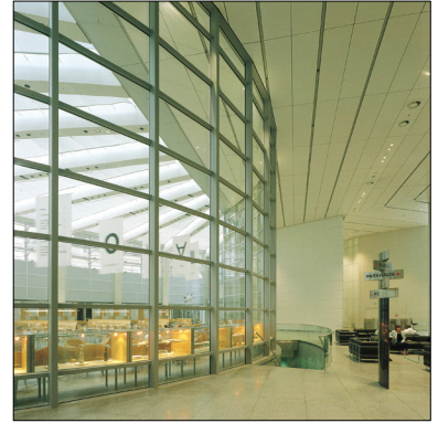
An example of internal fire-resistant partition.
