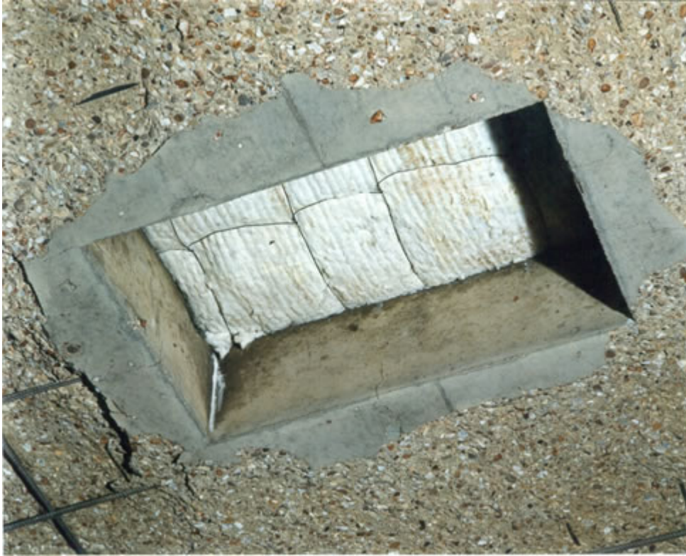
Figure 19 Picture showing spalling around service hole
