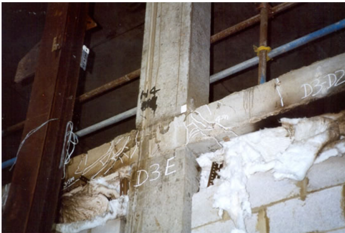
Figure 15 Cracking in the proximity of column D3
