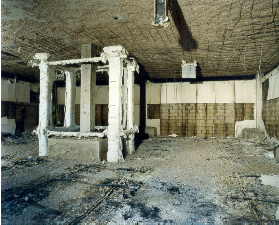
Figure 17 Picture looking into compartment from column D2 showing extent of spalling.
