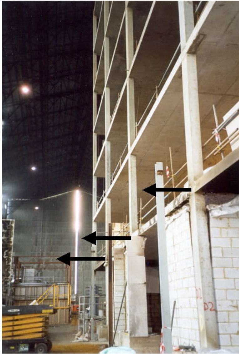
Figure 13 Picture showing lateral displacement of external columns.
