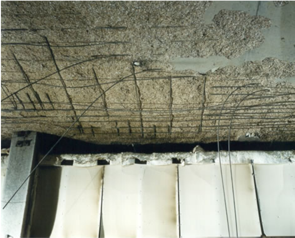
Figure 8 Picture looking at column C2 showing spalling to soffit of slab (Note: Failure of blanket fixings into slab soffit)
