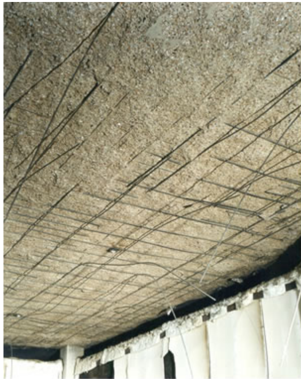
Figure 18 Picture showing spalling (looking at column B2)
