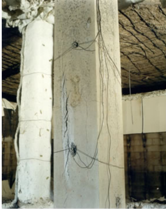
Figure 21 Longitudinal cracks in Column C3.
