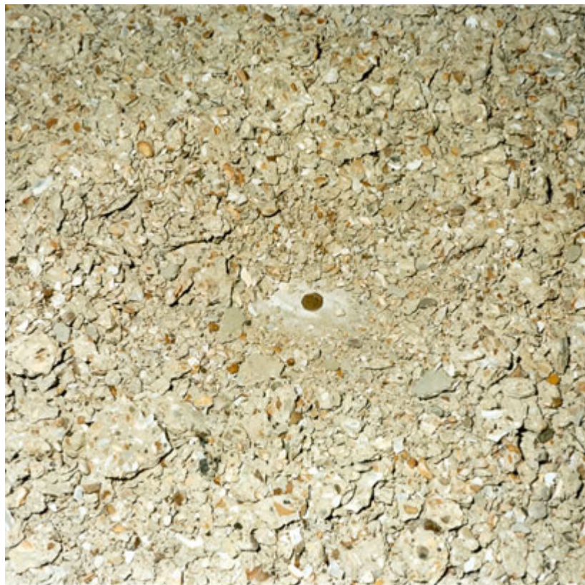
Figure 20 Picture showing extent of spalling (debris) on compartment floor (50 pence shown for scale)
