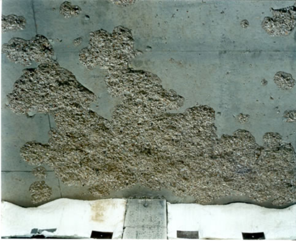
Figure 9 Picture looking at column D3 (Note: Fixings between blanket and soffit are intact due to limited spalling)
